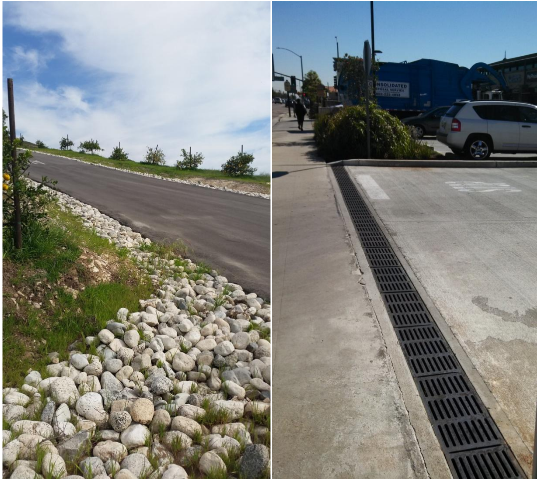
Figure 5: Infiltration trench (Rancho Palos Verdes, CA – Left; Seal Beach, CA - Right).
